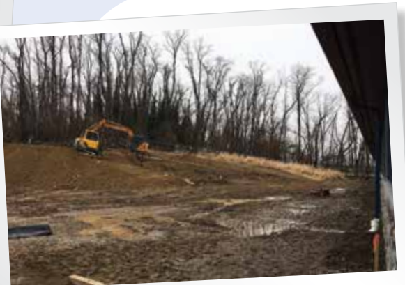
Construction crew cuts into our back hillside to level ground for the middle school
